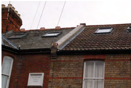
Example of unsympathetic concrete tiles and modern roof lights
