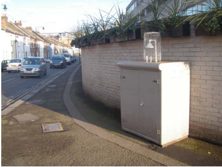
Figure 2.2 TRL monitoring station in Arthur Road
